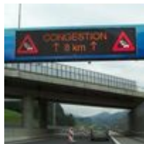
Variable message signs VMS LED
