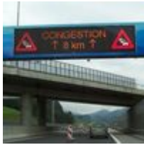
Variable message signs VMS LED
